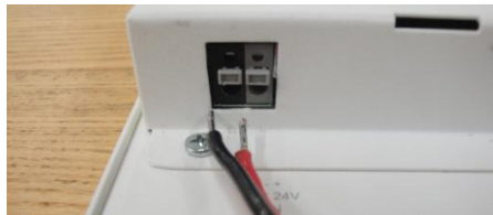
Fig. 10. Power to Terminal Block
